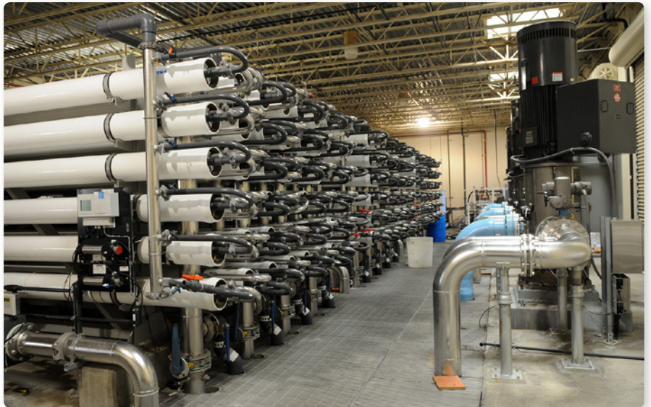
The Arlington Desalter provides a reliable high-quality water source.
